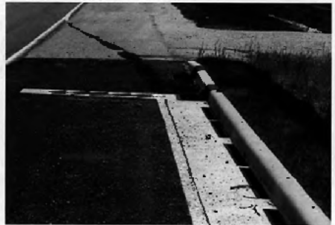
Rural Indiana where the Slotted Vane Drain is used to prevent recurring bank erosion. The design required a facility with high hydraulic capacity and low maintenance. The Slotted Vane Drain was installed parallel to the curb as well as perpendicular to the grate at the base of the hill to capture all the flow.
