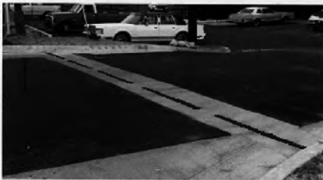
Installation in Tucson, Arizona employing the Slotted Vane Drain to capture runoff from the street; preventing flooding of the business, which is located at a lower grade than the street.
