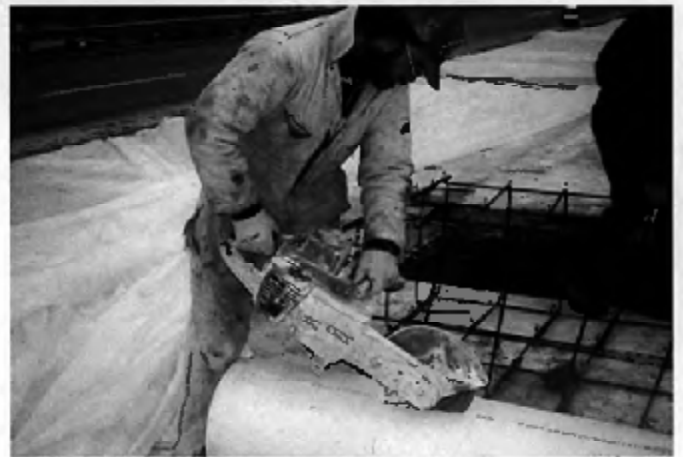
Construction techniques used in Wisconsin, utilizing a concrete saw to cut the top of the pipe and securing the unit prior to placing the concrete.
